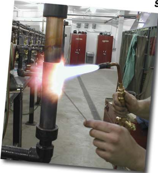
With more BTUs in the secondary flame a natural gas flame heats a joint more evenly and completely for better quality brazing
